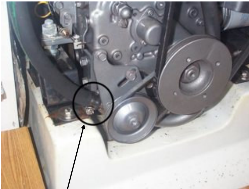
Location of hose that came off engine
