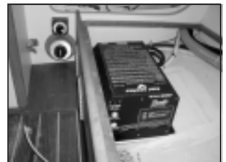
Freedom 10 inverter/charger under port settee
